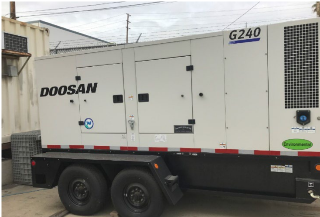
200 kW generator owned by the City of Long Beach, one of twenty-three such generators purchased collectively by the Cities of Long Beach and Los Angeles with FEMA funds.
