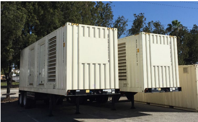
Two 800 kW generators owned by the LAC EMS Agency that are part of the fleet of twelve such generators purchased collectively by LAC and the City of Los Angeles using FEMA funds.
